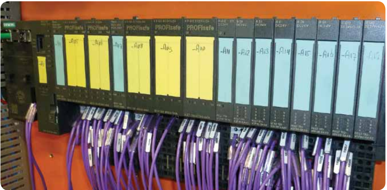
THE IMAGE ABOVE SHOWS THE SIMPLICITY OF THE NEW AS4024 COMPLIANT SAFETY CONTROL SYSTEM
